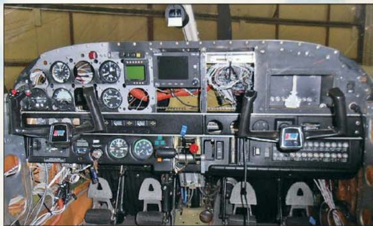
When its current upgrade is completed, Nolan Avionics' demo panel will include: Ultra Electronics AuRACLE CRM2100 engine monitor; PS Engineering PMA8000 audio panel; dual Aspen EFD 1000 PFDs, Aspen EFD 500 MFD, dual Garmin GTN 650s, GTX 327; Century Triden autopilot; and more.
